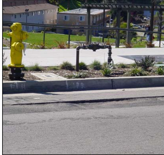
Poor trench repair at University Ave. and 52 nd St.
